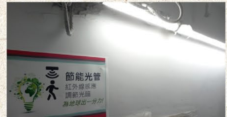
Site LED lighting with motion sensor
