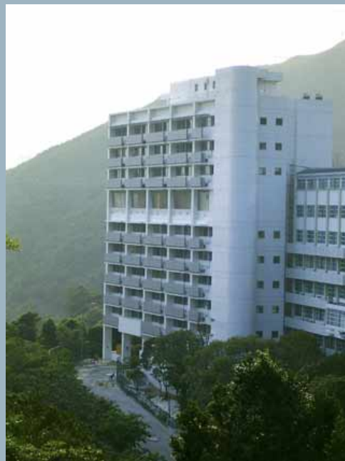
香港仔英基學校協會之學校擴建工程 School extension works for the English Schools Foundation at Aberdeen
